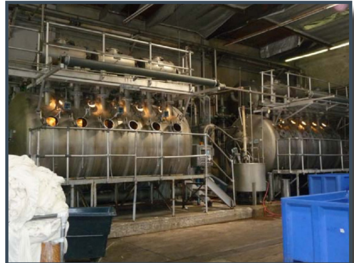
Building II: Fabric dye and boiler units
